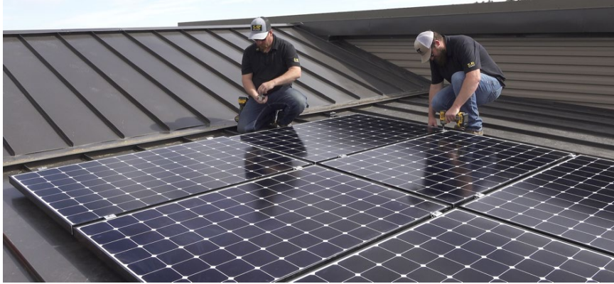
Figure 6: Solar PV Installation on Standing Seam
