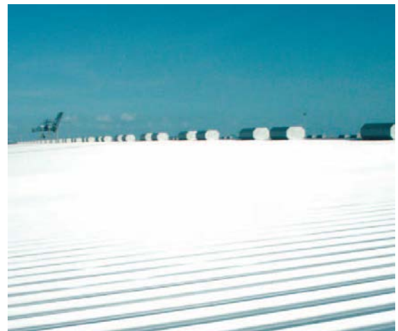
▲ Concealed fastened panels eliminate most fasteners from the weathering surface by using attachment clips inside the side-seam joint. The clips permit thermal movement, but because the “flat” of the panel is unrestrained, wind resistance is diminished. Under excessive load, the panel flat arcs upward, rotating the seam and disjoining.
